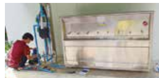
Installed Water Purifier and Water Fetching Place
